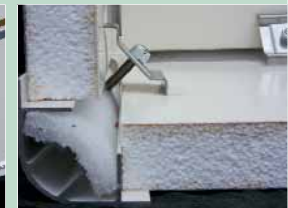
An early experiment shows how the panels are secured before a capping is added
